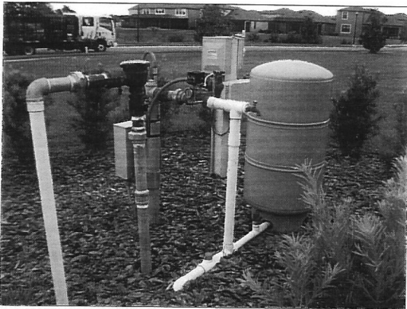
Well Pump and Holding Tank
